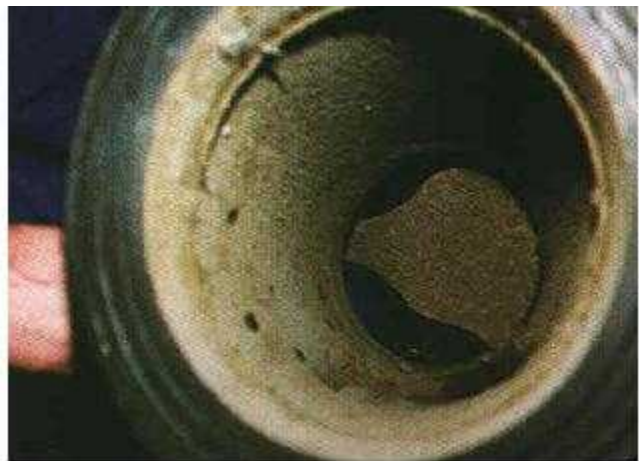
III.: The same muddy water pipe one year later on the inductive magnetic impact through the FLUID-LINER ®
